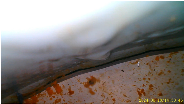
Figure 5: Water leak from klystron magnet.
