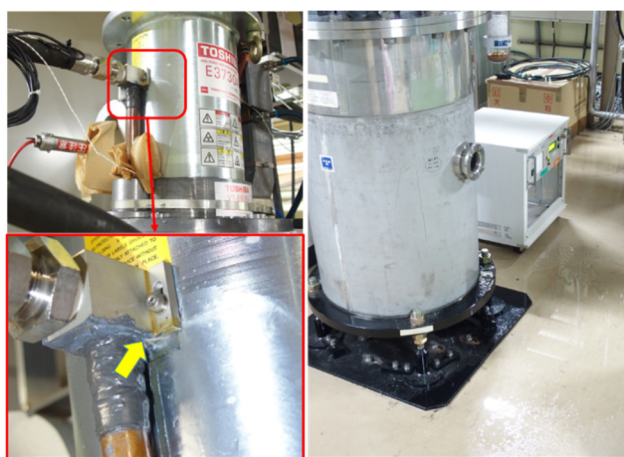
Figure 3: Klystron (C3) water leakage point.
